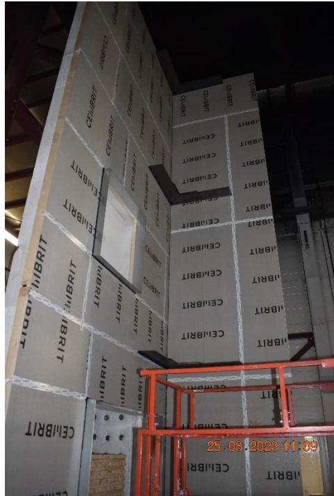
Photo No. 5 Steel profiles around window and fire chamber has been installed.
