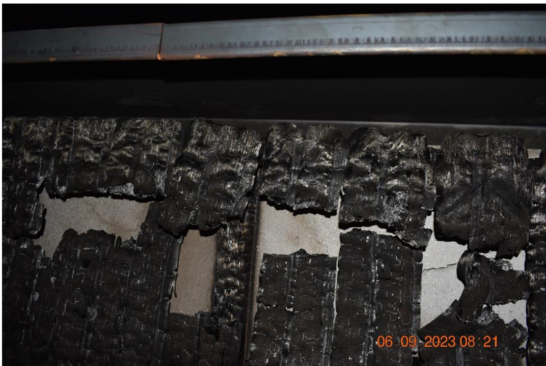
Photo No. 24 Test specimen after the test. Detail photo of cladding above the fire chamber.
