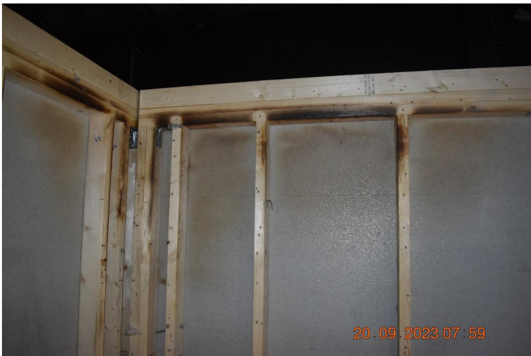
Photo No. 32 Construction wood in the top corner.
